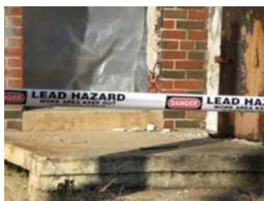
"Danger: Lead Hazard" tape stretched across a work area.
